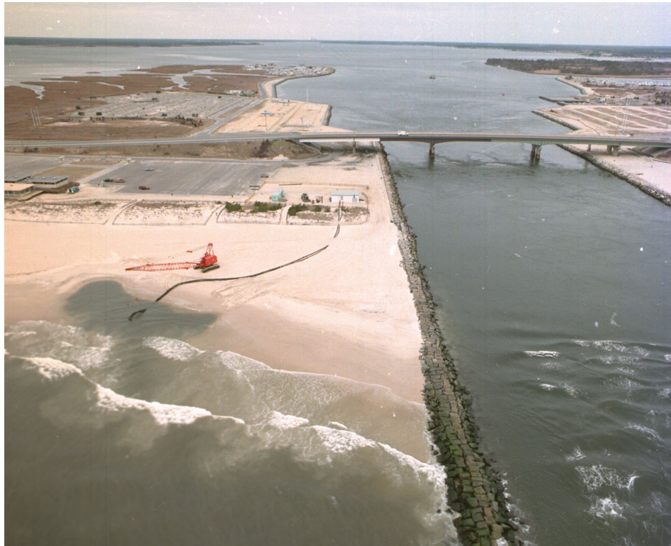
Figure 2-21. Indian River Inlet Sand Bypass System (USACE, 2020)
